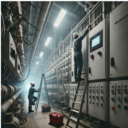
Poor or limited location makes equipment difficult to maintain.
